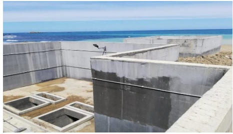
d) El Marsa station pumping basin
