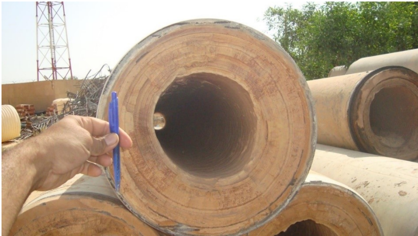
Figure 21: The condition of the drinking water supply network pipes in the town of Touggourt after 7 to 8 years of service (Photo Remini, 2016)
