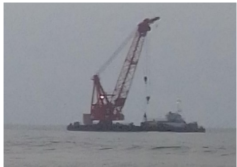
b) Laying the raw water collection pipe from the Corso desalination plant
