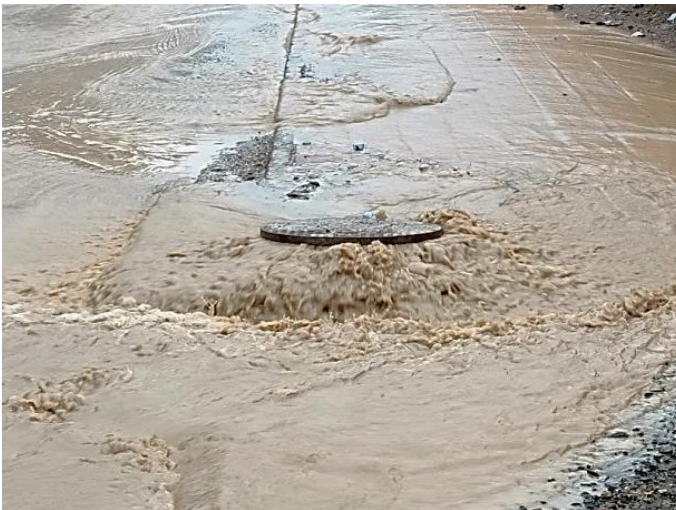
Figure 29: Sanitation networks are today undersized in the face of the flash floods occurring in Algeria (Photo. Remini, 2023)
