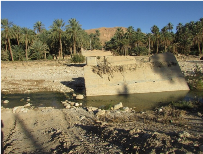
Figure 11: A bridge crossing the Labioid wadi to reach the village of Mchouneche was swept away by the flash flood that occurred from October 28 to 31, 2011 (Photo. Remini, 2011)
