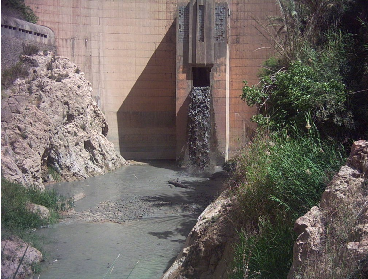
Figure 19: Under the effect of the vortex, caused by the opening of the valve for withdrawing the density current, a palm tree obstructed the closing of the bottom valve of the Fom El Gherza dam (Biskra) in 2006 (Photo. Remini, 2006).
