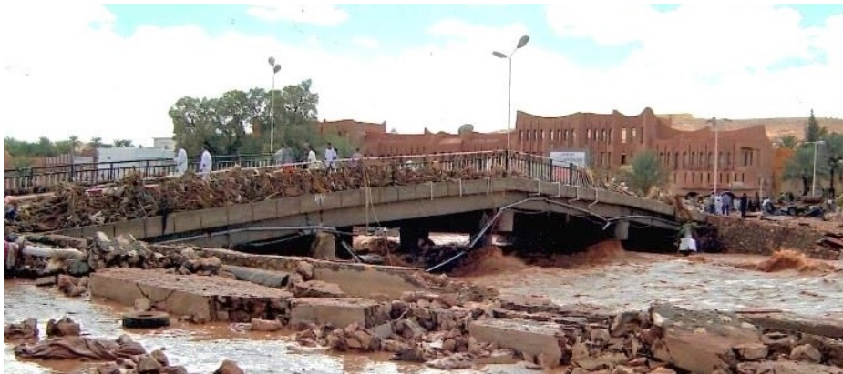
Figure 14: Floating objects formed a temporary barrier on the bridge in downtown Ghardaïa (Photo. Heritage)
