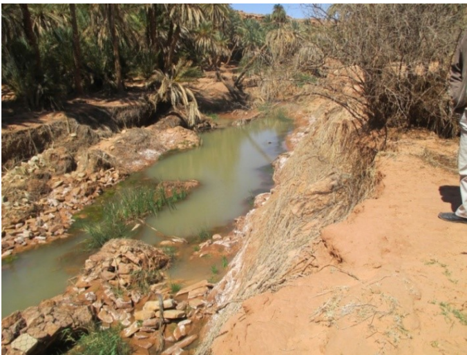
Figure 13: The banks of the wadi were eroded by flash floods that crossed the Asla oasis (Photo Remini, 2012)
