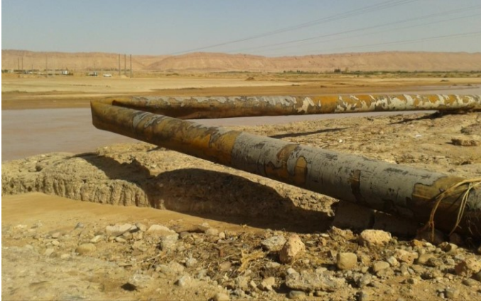
Figure 9: M’Zi River– Flood of September 30, 2016. Shearing of the pipe (Photo. Sonatrach, 2016)
