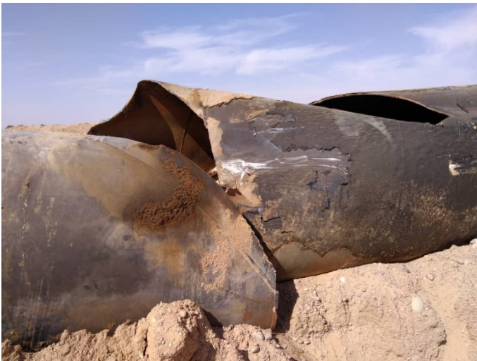
Figure 10: Ittel River- Saharan Flood of September 3, 2020. Brutal shearing of the pipe. (Photo. Sonatrach, 2019)
