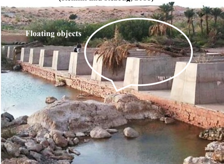
b) New weir barrage constructed at the end of the Ninety (Remini and Rezoug, 2018)
