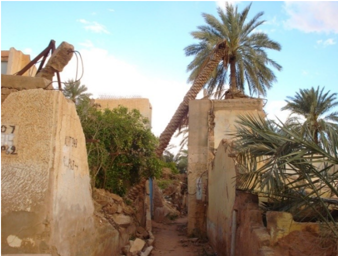
Figure 6: Damage caused by the passage of the flood on October 1, 2008, in the Wadi of Mzab (Photo. Remini, 2008)
