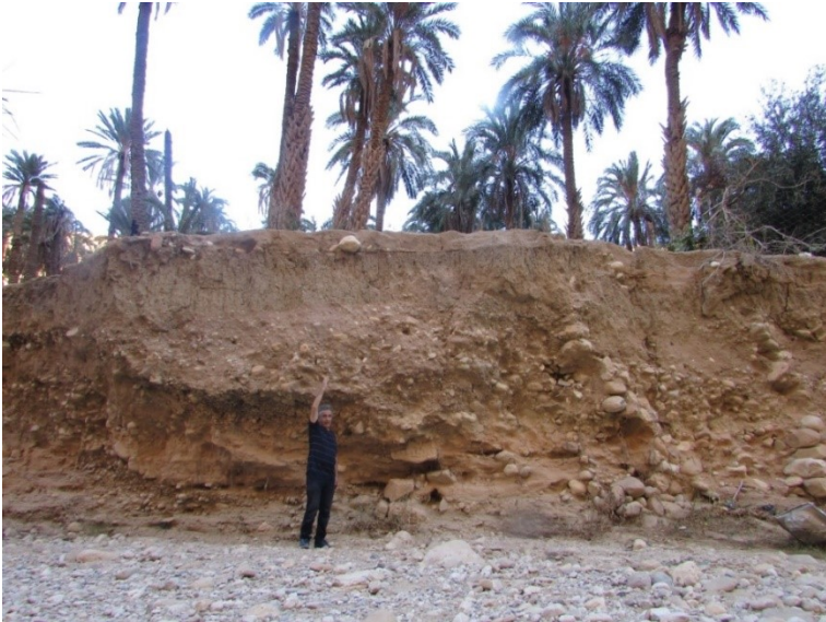
a) Undermining of the banks in Wadi of Labiod (Photo. Remini, November 2023)
