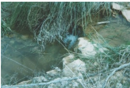
Photograph 2: Water leaks on the left bank next to the SB13 piezometer at Ouizert Dam (Benfetta, 2018)
