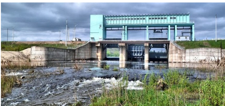
Figure 3: Operation of the constructed spillway of the first stage with two outer spans.
