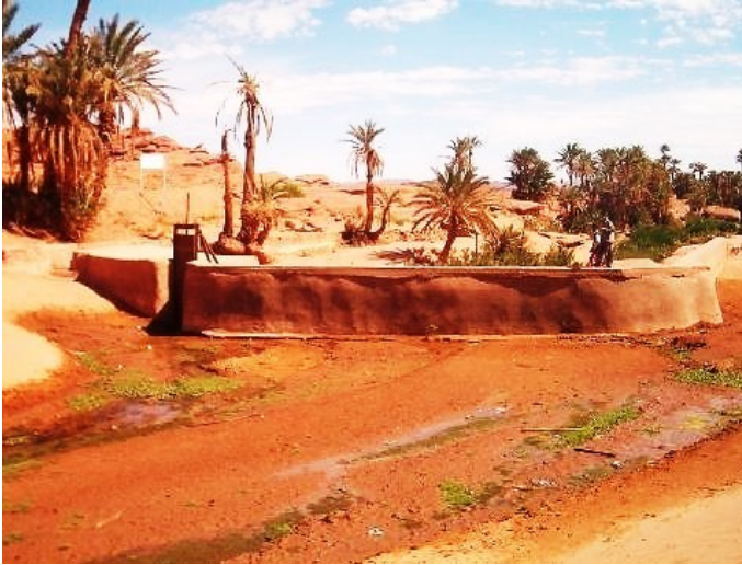
Figure 1: Tiout Dam, among the first dams built in Algeria (more than 7 centuries) (Photo. Remini, 2006)
