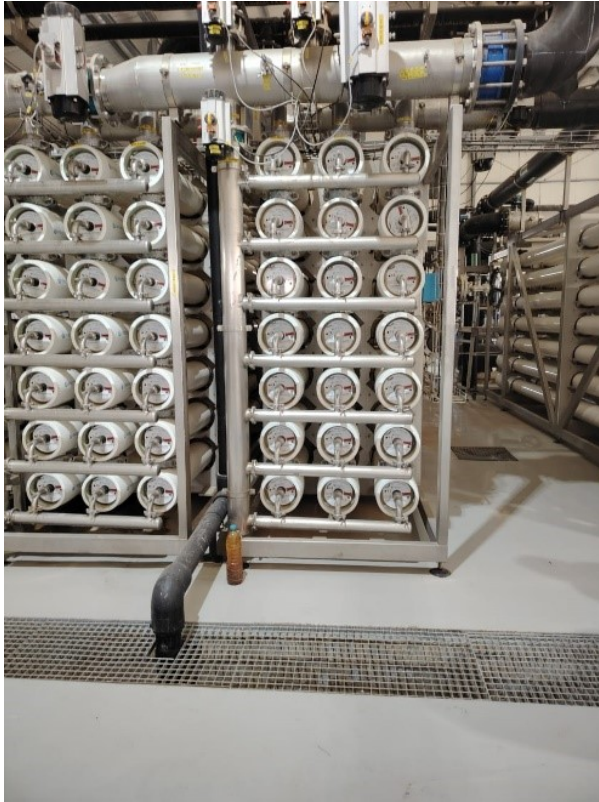
Figure 9: A brackish water desalination plant in southern Algeria (Photo Remini, 2024).
