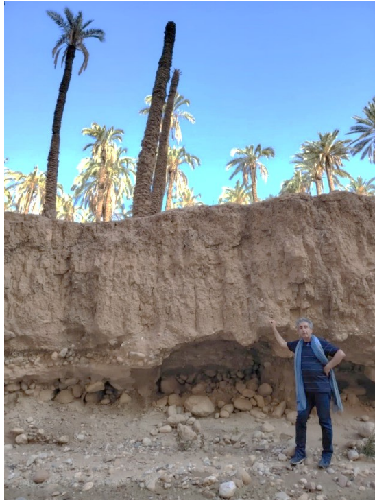
Figure 7: The importance of the undermining of barges at the level of the Labiod wadi having an impact on the silting of the Foum El Gherza dam (Photo Remini, 2024).
