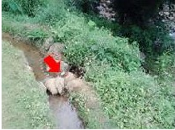
Image 5: Spillways with breakable weirs
