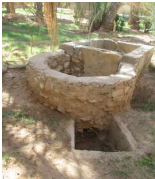
Figure 39: Recharge well in the El Guerrara oasis equipped with an opening to allow floodwater to fill the well (Photo. Remini, 2014)
