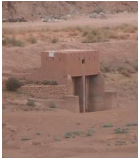
Figure 42: Drain valves from the Bouchen dam (Photo. Remini, 2016)
