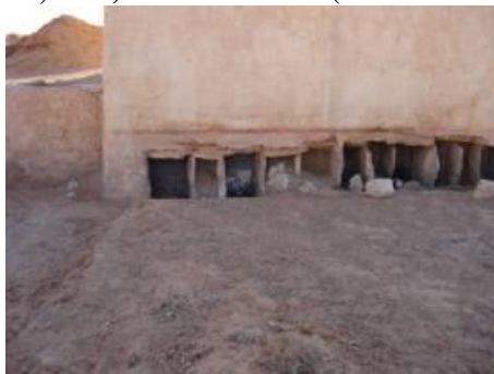
Figure 27: Drainage which allows water to flow into the Tardja N'Takdimt (Photo. Remini, 2014)
