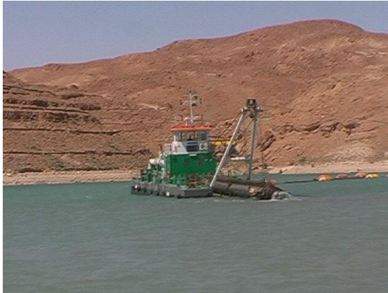
Figure 9: Dredging operation in the Foug El Gherza dam (Photo. ANBT-Foug El Gherza Dam)
