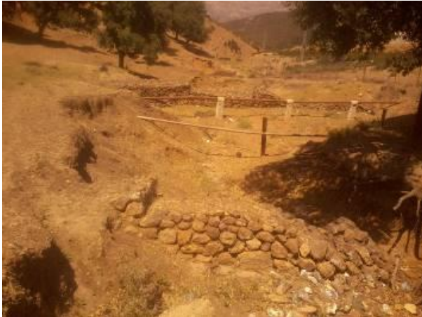
Figure 15: Torrential correction by gabions in the watershed of the Zardezas dam, Algeria (Photo Toumi, July 8, 2015)
