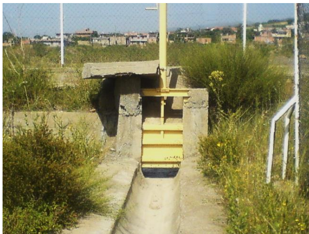
a) Water intake from the El Harrach River
