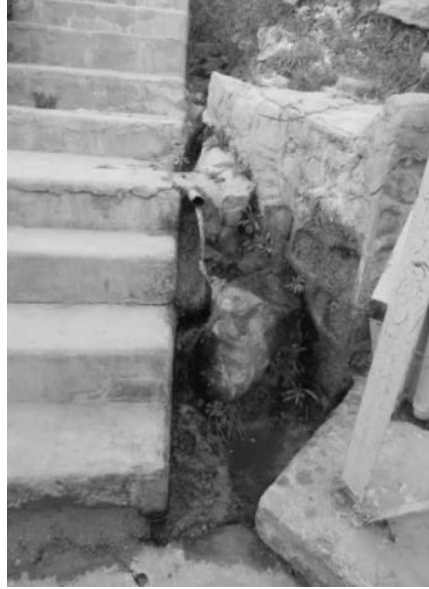
Figure 14: Water leak at the left bank of the dam Foum El Gherza (Photo. Remini, 2016)
