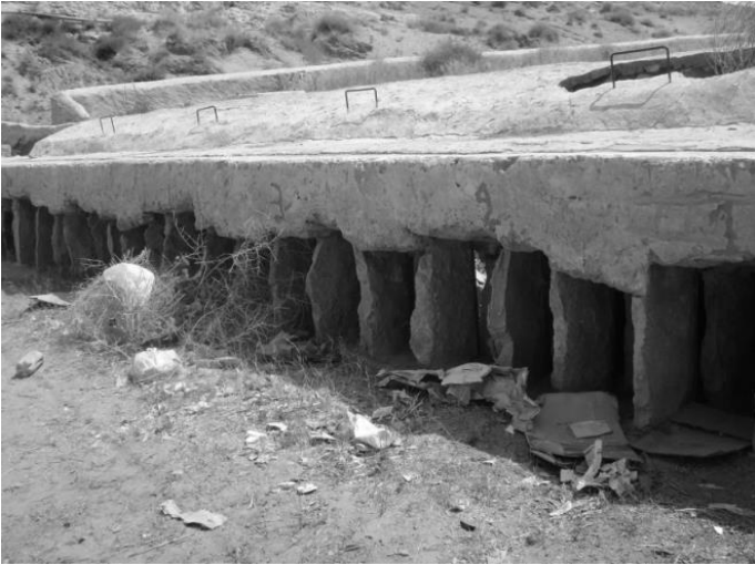
Figure 18: Tissanbadh of the water distribution network of the oasis of Ghardaïa (Photo. Remini, 2008)
