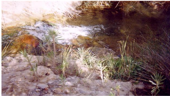
Photograph 2: Water leaks on the left bank of the Algerian Ouizert Dam. Source: Benfetta, 2021.
