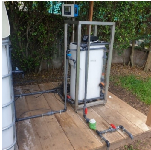
Figure 3: Water denitration pilot unit
